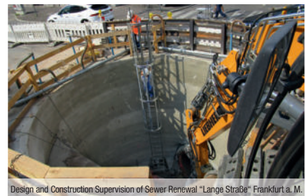
Design and Construction Supervision of Sewer Renewal "Lange Straße" Frankfurt a. M.
