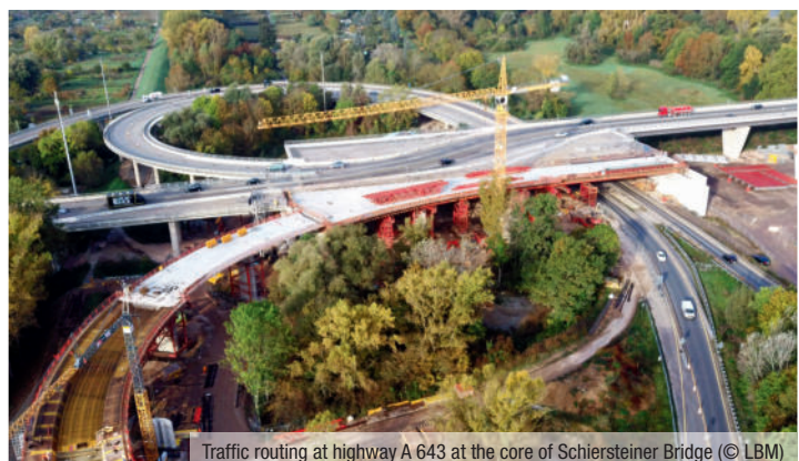
Traffic routing at highway A 643 at the core of Schiersteiner Bridge (© LBM)
