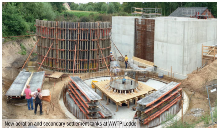
New aeration and secondary settlement tanks at WWTP Ledde
